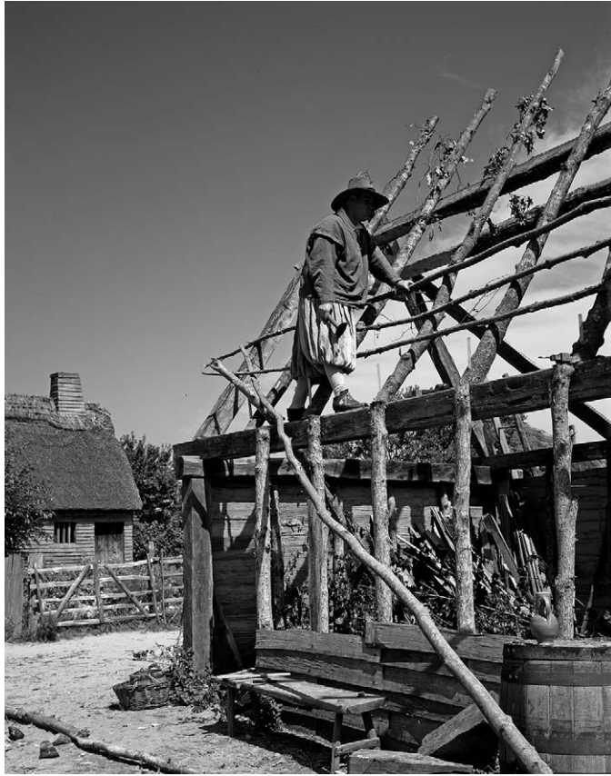
Building a house at Plimoth Plantation, 1980. (Carol M. Highsmith Archive, Library of Congress, Prints and Photographs Division).
